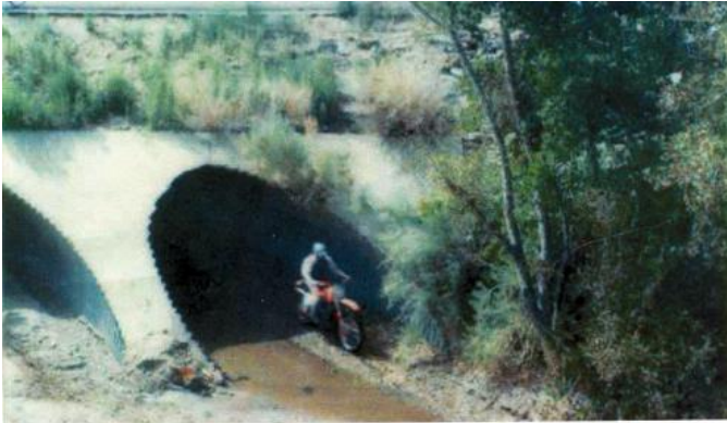
CYC Access Road Culverts circa 1978 -- wash silted in more than 8 feet
