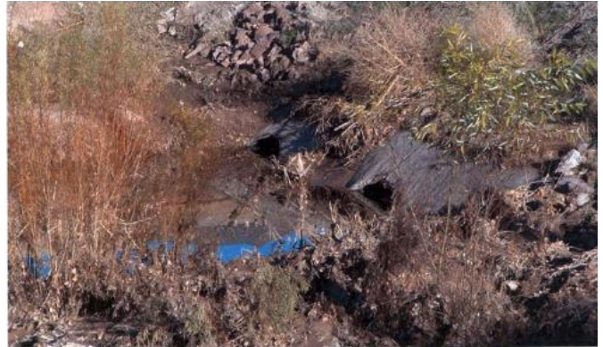
CYC 12 Foot Culverts -- downstream side showing depth of sedimentation 11/19/2004
